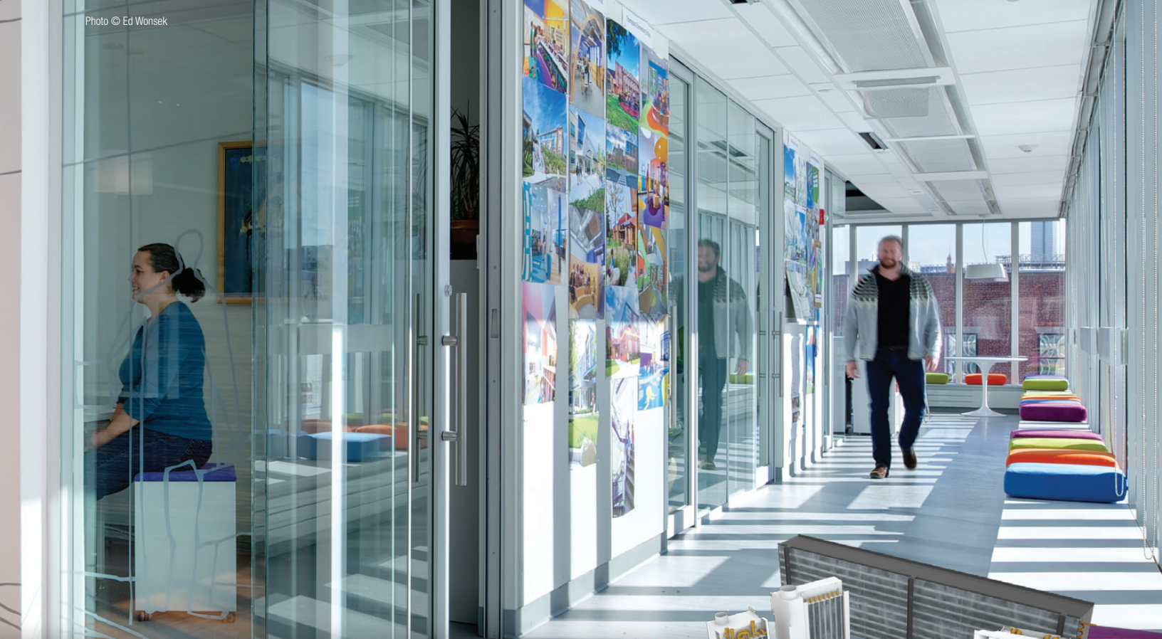
Above: Chilled Beams
